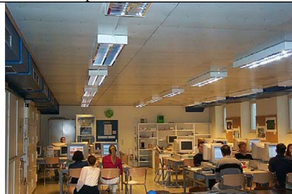
Measure 7 and 9: Ventilation installation computer room: Switch off ventilation completely if possible, windows are existing. (...) If fresh air operation necessary, stage 1 sufficient. Check ducts: supply air outlet barely perceptible, although air change of 3,600 m 3 /h is set.
