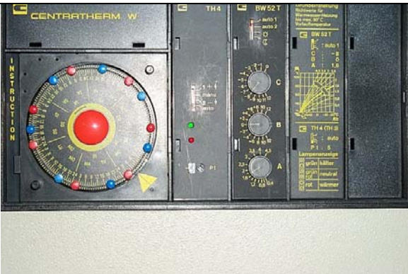
Measure 3: Adjustment of heating times to utilization: Switch off Sa + Su, postpone start of heating-up operation Mo – Fr from 2, 3 and 4 o'clock respectively to approx. 5 to 6 o'clock.
