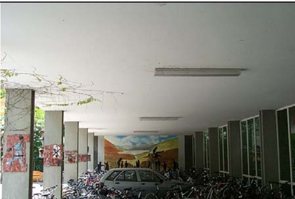
Measure 2: Insulation of the floor slab against ambient air. Comfort problems in relevant rooms.
