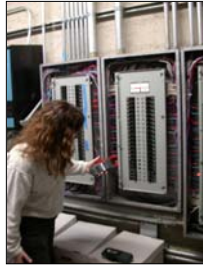
Measuring power at the panel
