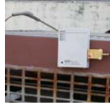
Measuring flue gas temperature
