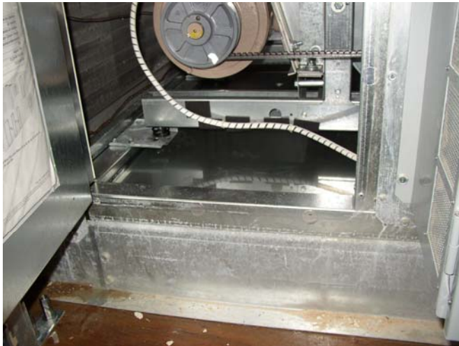
Figure 2—That reflection in the AHU basin is not shiny metal. It's standing water that won't drain if the pan is sloped away from the drain!
